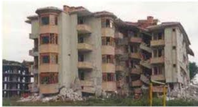
Figure 1. Irregular shape structure disaster
